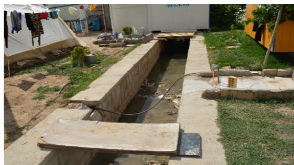
Figure 18. Clogging of water in canals (Source: Authors)
